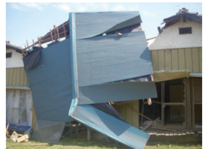
Photo 3: Impact from flying debris (roof)
