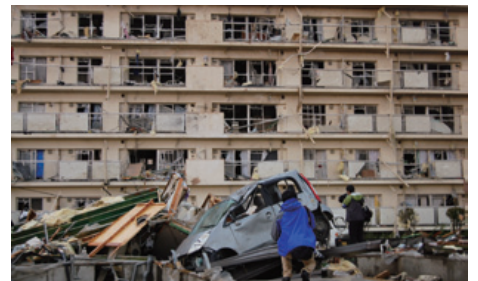
Photo 5: An apartment building with extensive damage to non-structural elements
