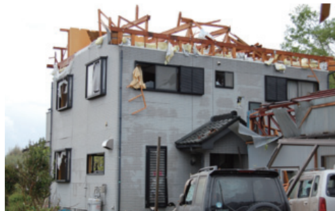
Photo 2: Destruction caused to a wooden house
