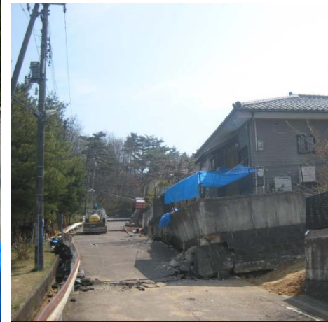
Damage of retaining wall and house movement
