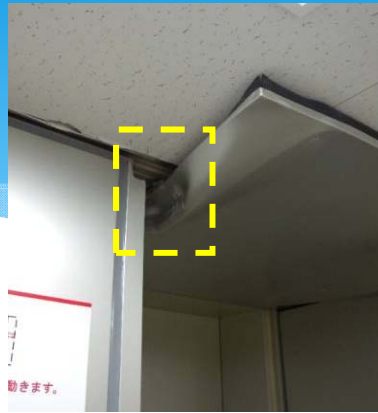
Damage to expansion joint
