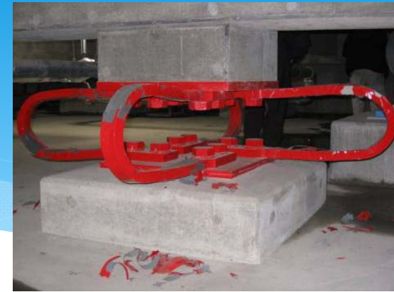
Peeled off of paint on U-shape dampers
