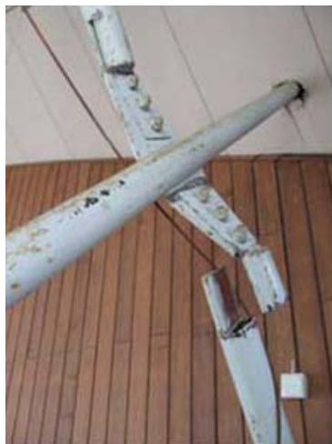
Rupture of brace at joint
