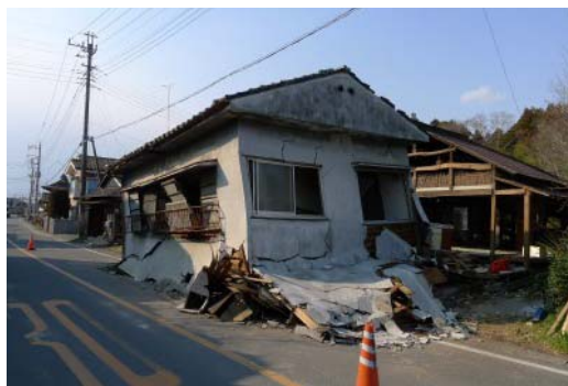
Collapse of 1 st story
