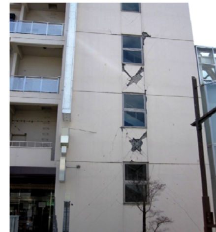
Shear failure due to opening of shear wall
