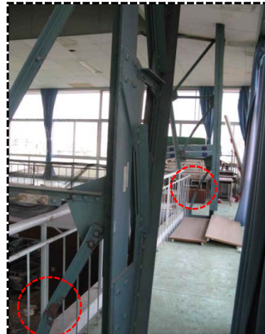
Buckling of diagonal member of latted column
