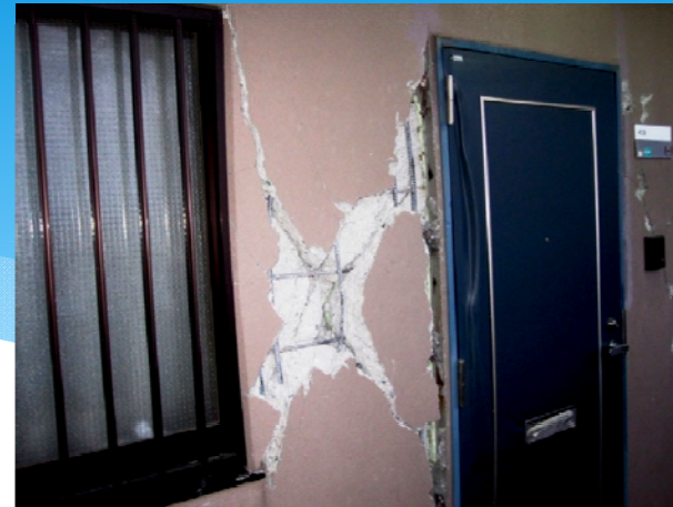
Shear failure of non-structural walls
