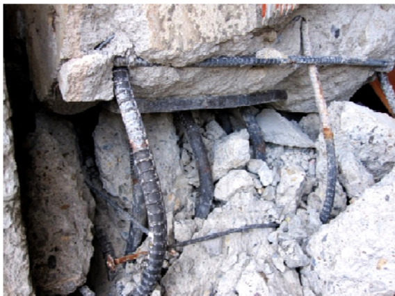
Pullout of anchor bolts of the exposed-type SRC column base
