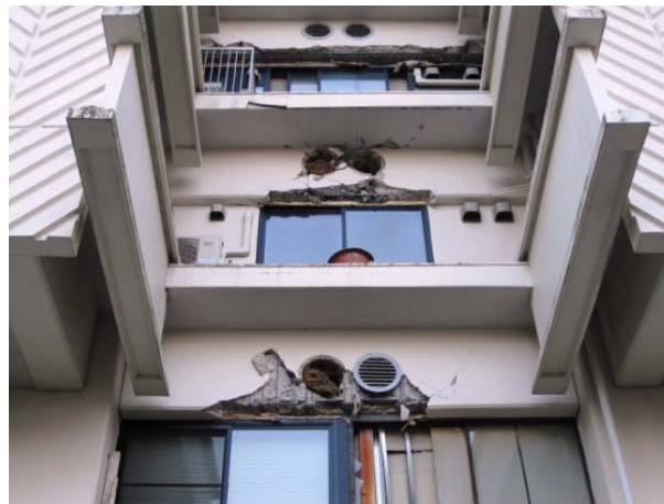
Shear failure of link-beam
