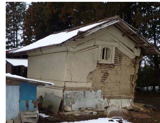
Damage of Dozo (Japanese traditional wood storehouse coated with clay and plaster finish)
