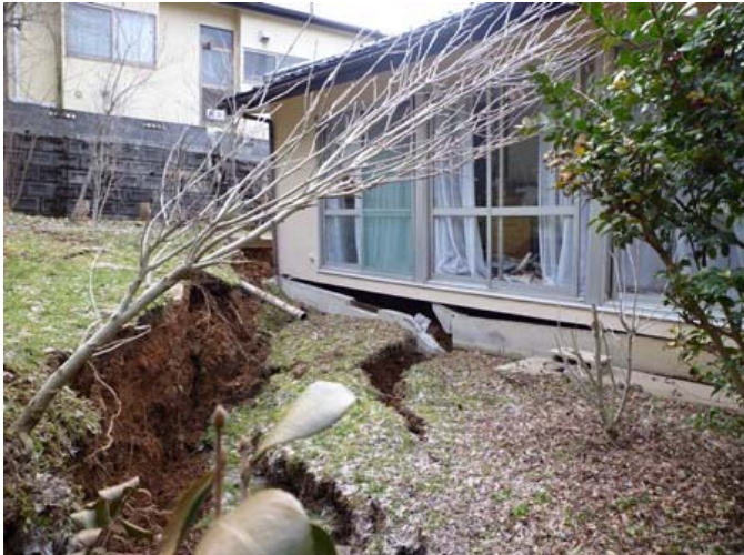
Failure of footing caused by the ground damage
