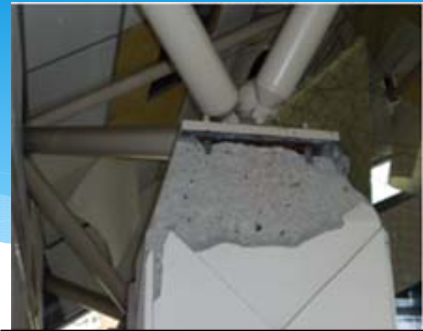
Spalling of concrete at joint
