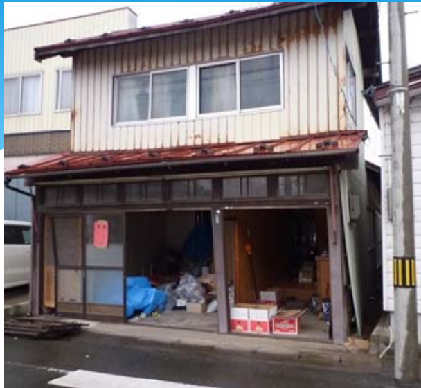
Damage of houses with store (Inclination of 1 st story)
