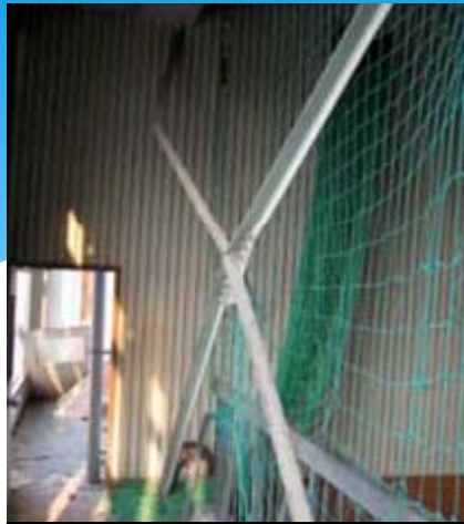
Buckling of brace
