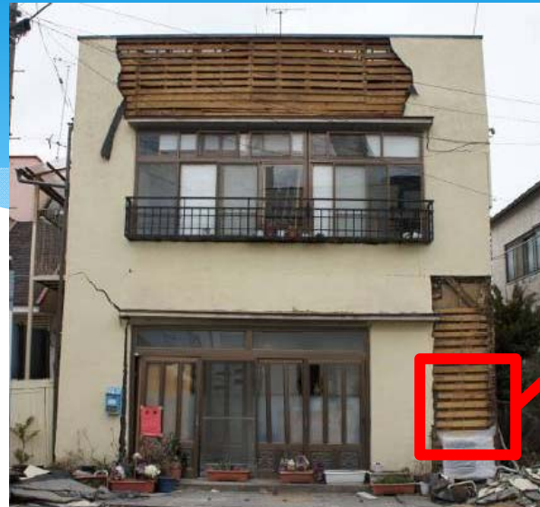
Damage due to Bio-deterioration
