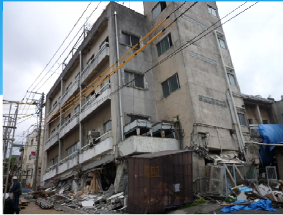
Collapse of soft-1 st story by shear failure of columns
