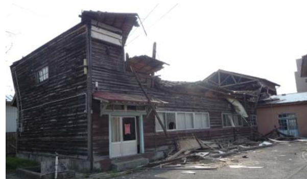
Collapse of 2 nd story
