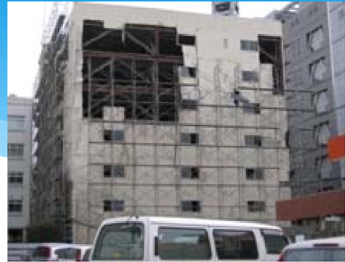
Fall of exterior wall panels
