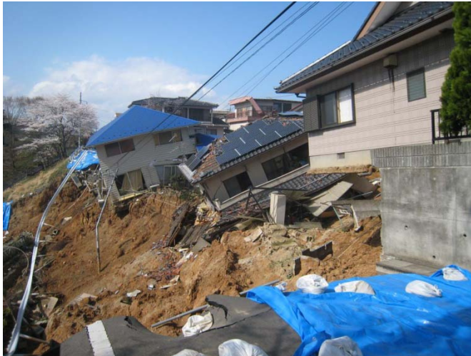
Land sliding on the slope of the developing hill
