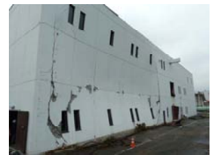
耐力壁の破壊
